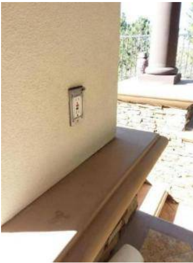
Photo 15-1 Outdoor room column - cover missing
