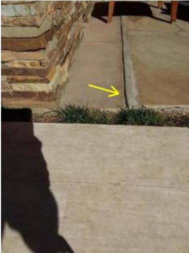
Photo 5-1 Elevation change in concrete slabs due to settling
