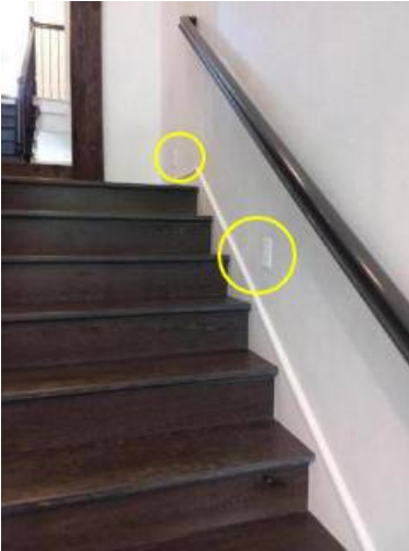
Photo 19-1 Stairwell wall lights
