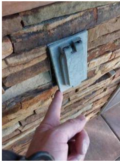
Photo 15-2 Near the BBQ area sink - loose
