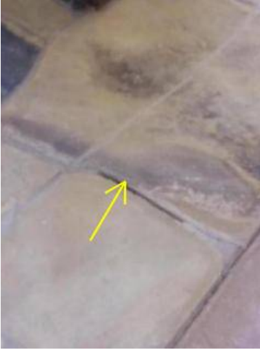
Photo 7-1 Grout missing in some areas of the patio flagstone
